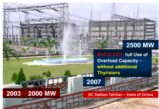
Fig. 9: Site View of Indian East-South Interconnector – DC Station Talcher
