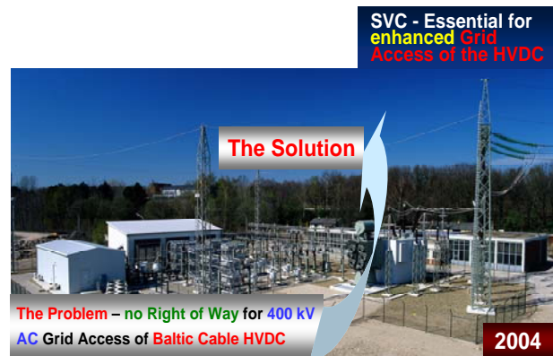
Fig. 14: The Solution – the first HV SVC in the German Grid at Siems Substation
